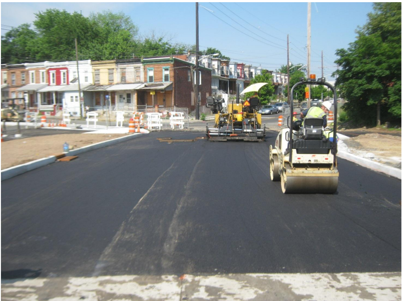
Shown above is the placement of asphalt for the pedestrian path at the east side of the pedestrian bridge (top left), the placement of asphalt for the easterly portion of the pedestrian path (top right), and the placement of asphalt for the west approach roadway (bottom).
