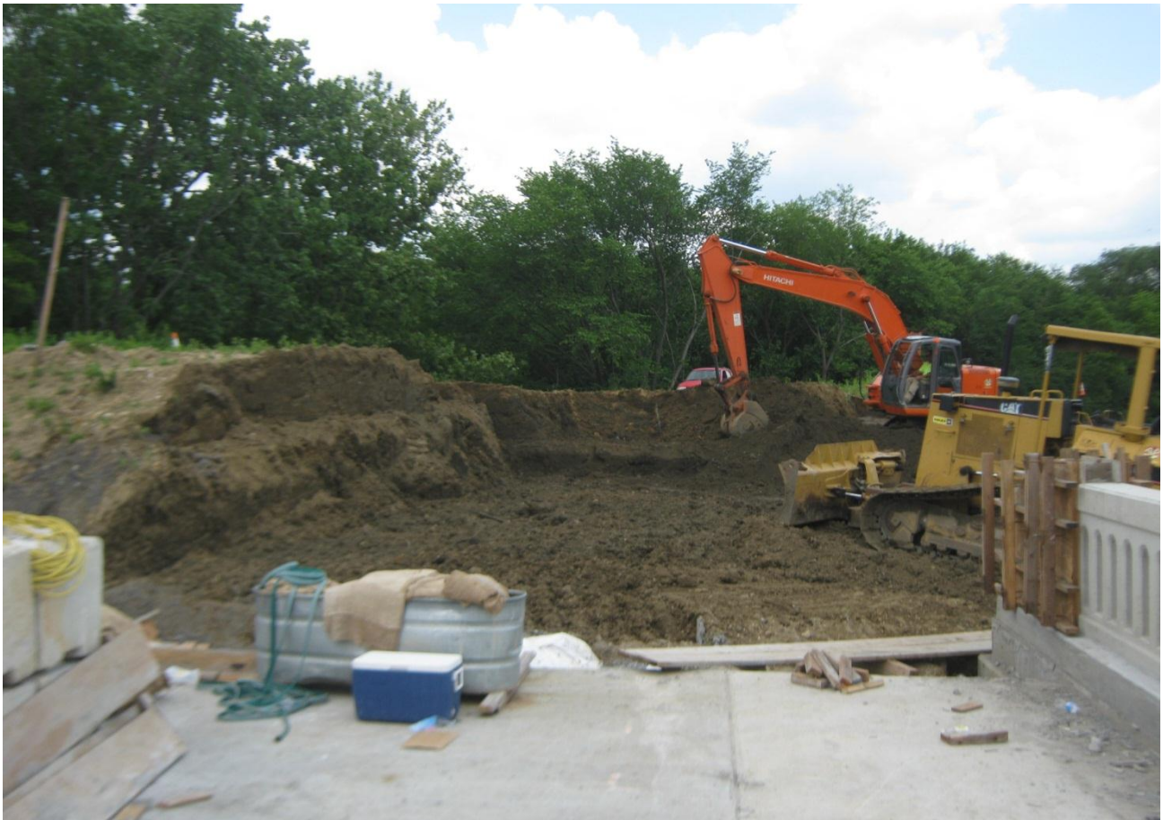
Shown above are images of the contractor beginning to remove the temporary surcharge material.
