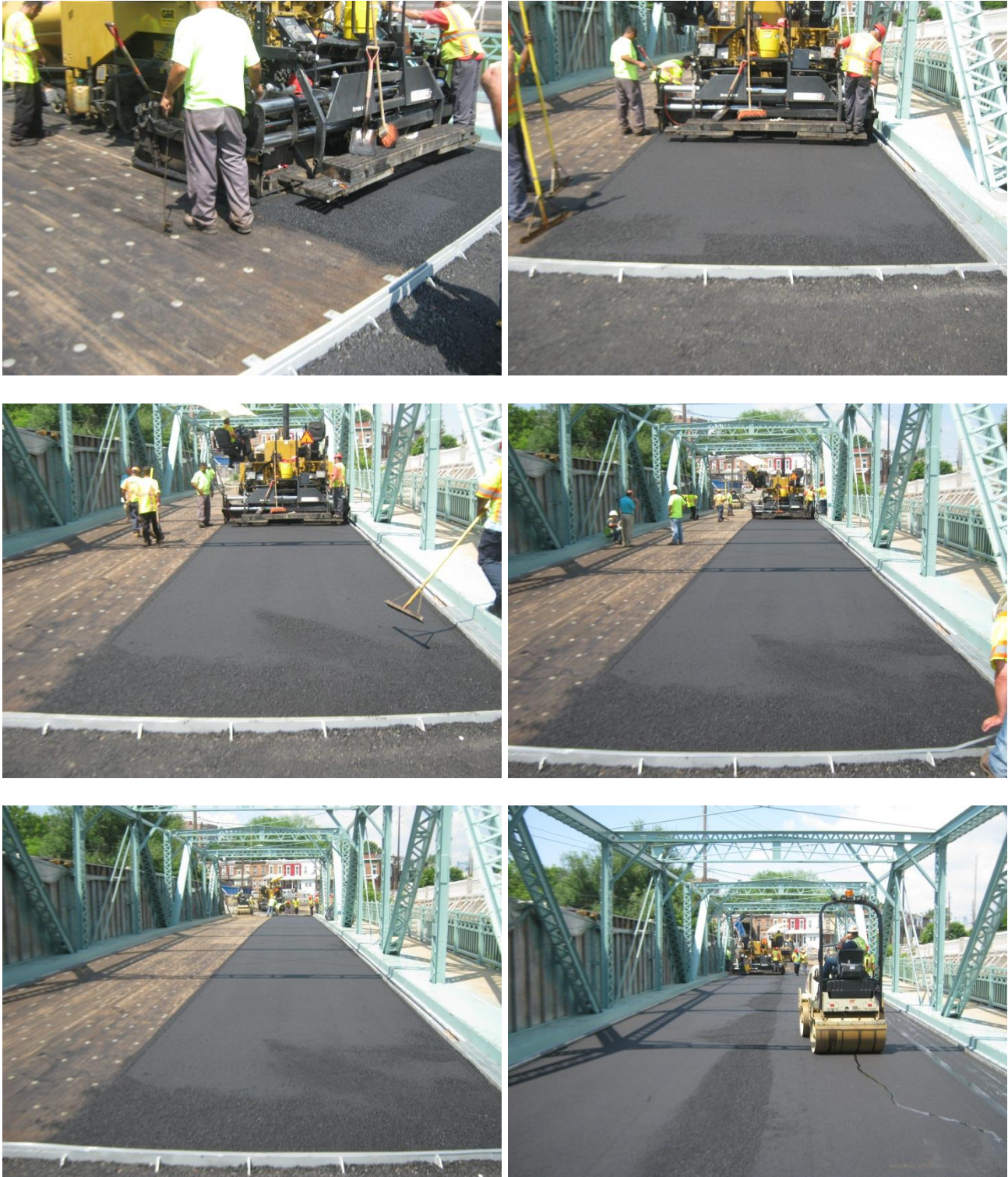
Shown above are images displaying the progress during the placement of the asphalt scratch course on the pedestrian bridge.
