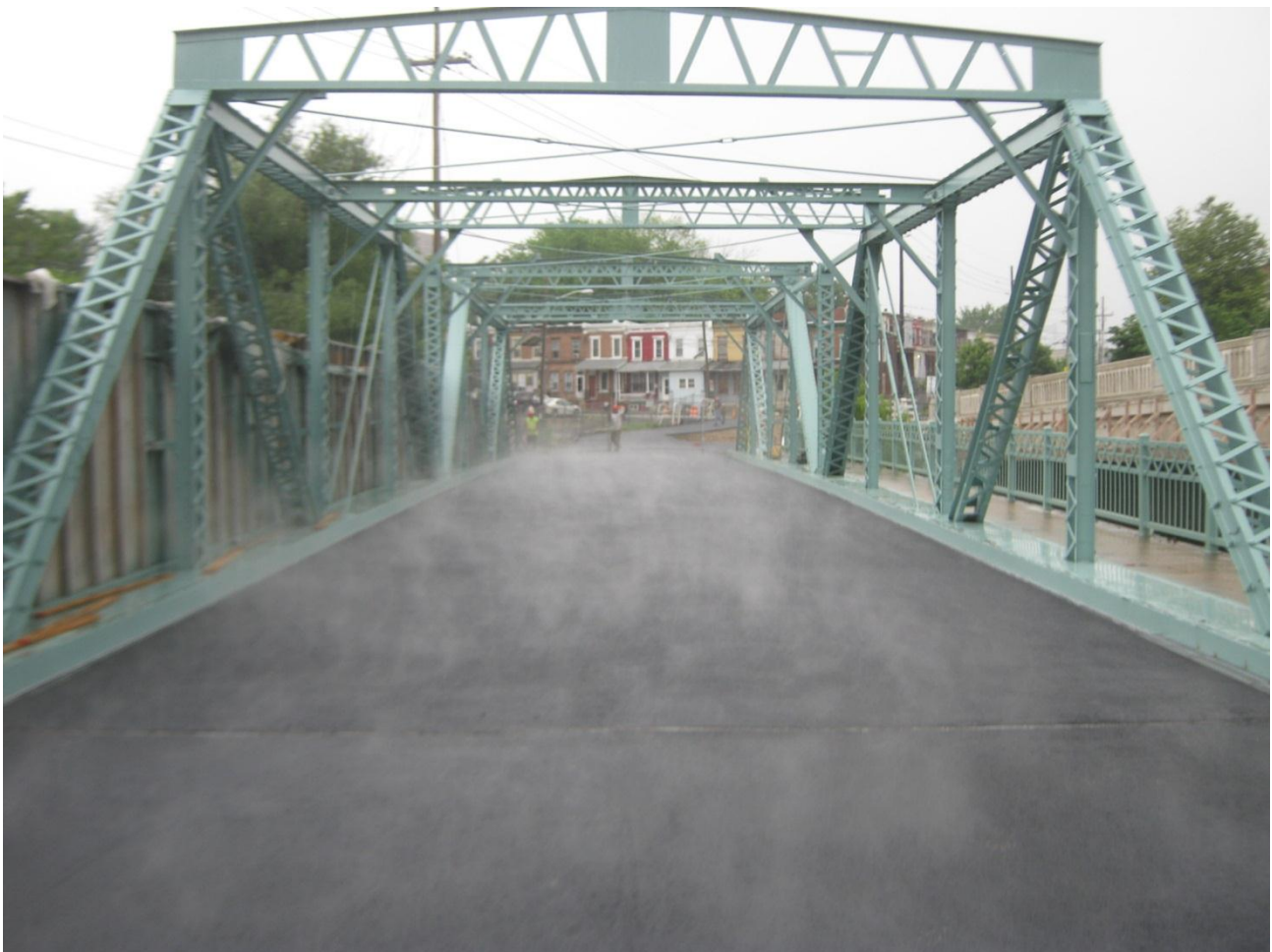
Shown above is the contractor installing the waterproofing membrane (top left), the placement of asphalt (top right), and the pedestrian bridge after the asphalt was placed and compacted (bottom).
